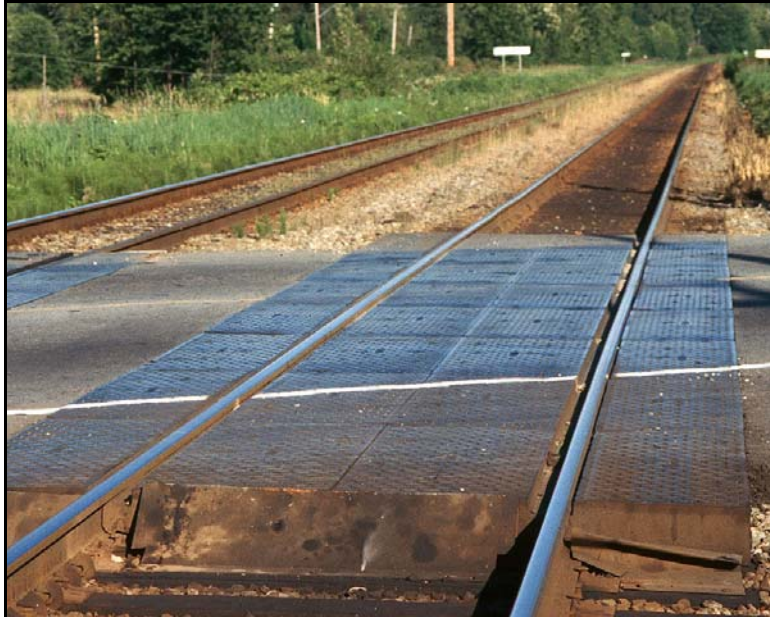
Figure 4.36 — Rubber track guard at railway crossing
