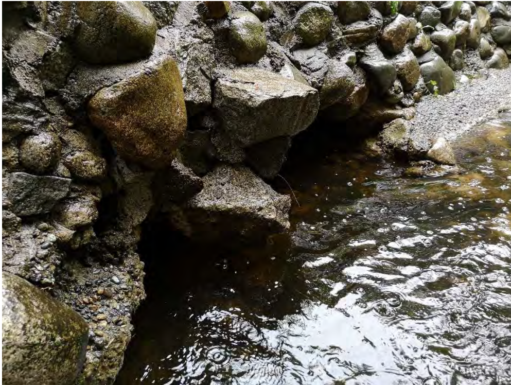
Figure 6. Rodgers Cr, scour observed along the left (northern) bank adjacent to the greenhouse - facing northeast
