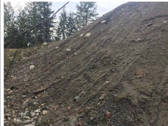
Photo 6. Exposed fill slope adjacent to and within the 30-m setback from Rodgers Creek top of bank; rilling soil erosion identified (2017.06.01).
