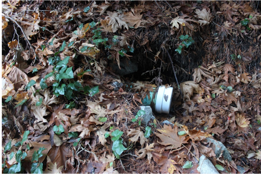
Photo 3. Sealed connection at drainage channel to DWV storm water utility.
