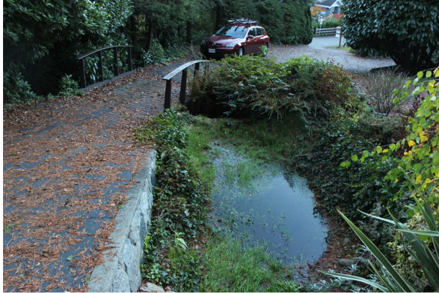
Photo 7. Manmade pond with concrete weir at wood bridge. Limited riparian area at rock wall/asphalt drive. View looking downstream towards Piccadilly Drive.
