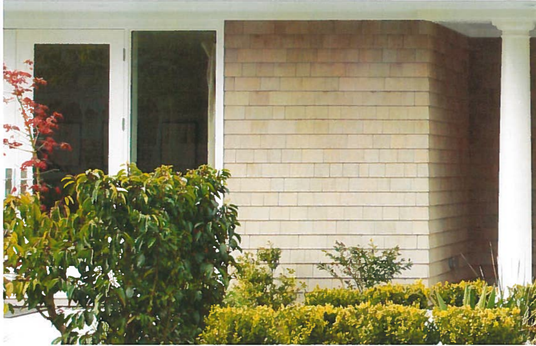
13 Wall shingles will be # 1 boxed "perfection" resawn and rebuffed Western red cedar shingles stained with General Paint "Glutted" colour semi-solid stain, 5" to weather. The roof will be quaternian treated resawn western red cedar, 5 1/2" to weather
