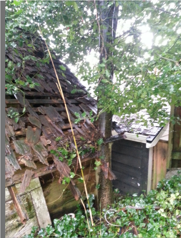
Photo 5. Tree # 5985 is growing through the existing carport roof.
