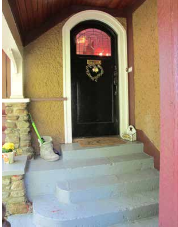
Existing entrance door above concrete stairs of entry porch. Note low stone balustrade and stained soffit beneath porch canopy.
