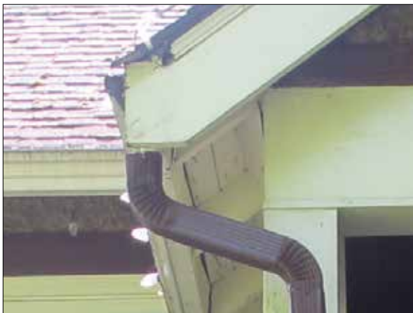
Cross-gabled roof structure of the Sutherland House (top); exposed roof rafters and nailing boards (middle); and typical condition of roof drainage (bottom)
