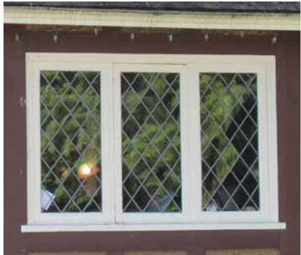
Typical condition of existing tripartite windows on the front facade to the north.
