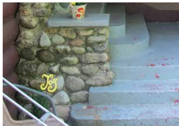
Photos showing typical condition of extant original side-entry porch and stairs of the historic house. Note the crack along the mortar, which also shows biological growth.
