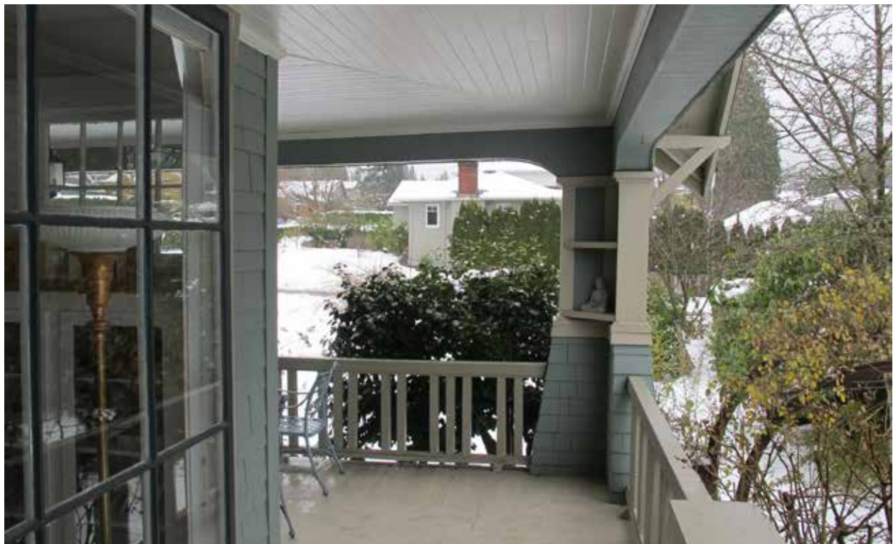
Photos showing existing condition of wrap-around verandah. Note the later porch-deck extension to the verandah (top, left)
