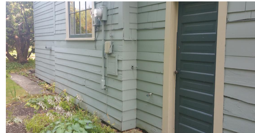
The pattern of cedar shakes and horizontal siding will be retained and replicated on the new Laneway and Garden Cottages
