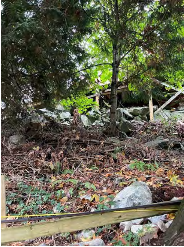
Figure 2: Insufficient Footings and Supports
