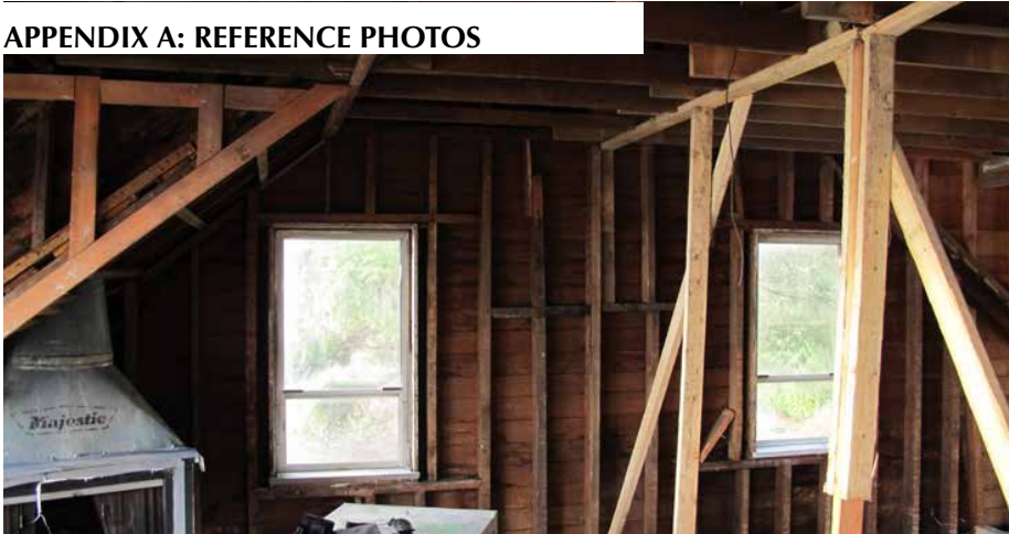
None of the window frames or assemblies have survived, but the window openings are clearly evident on the second floor and provide measurements for how the windows can be restored. Original double-hung configuration as per archival photos.
