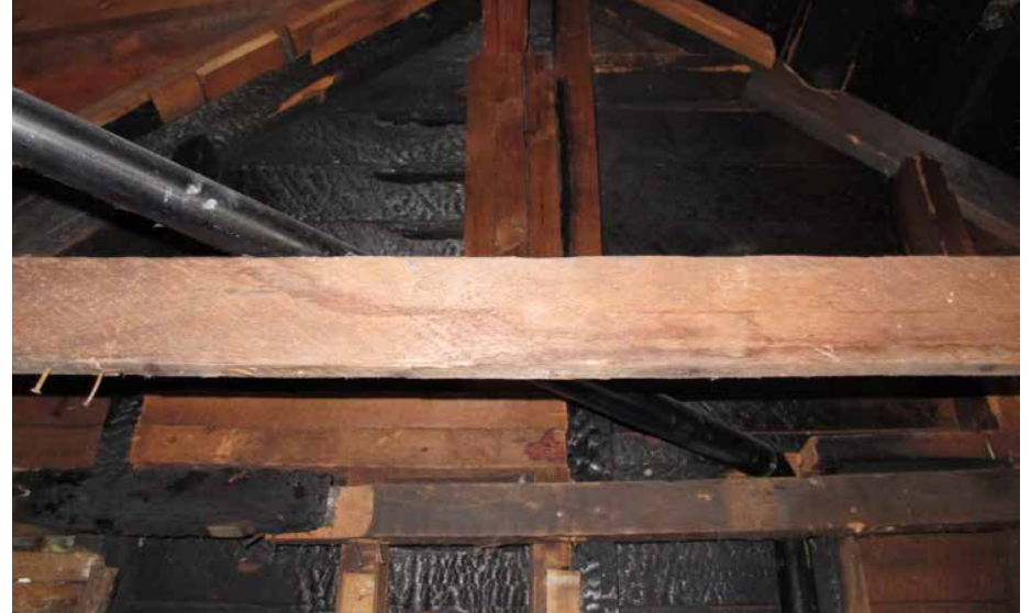
Evidence of chimney fire in the East Gables.
