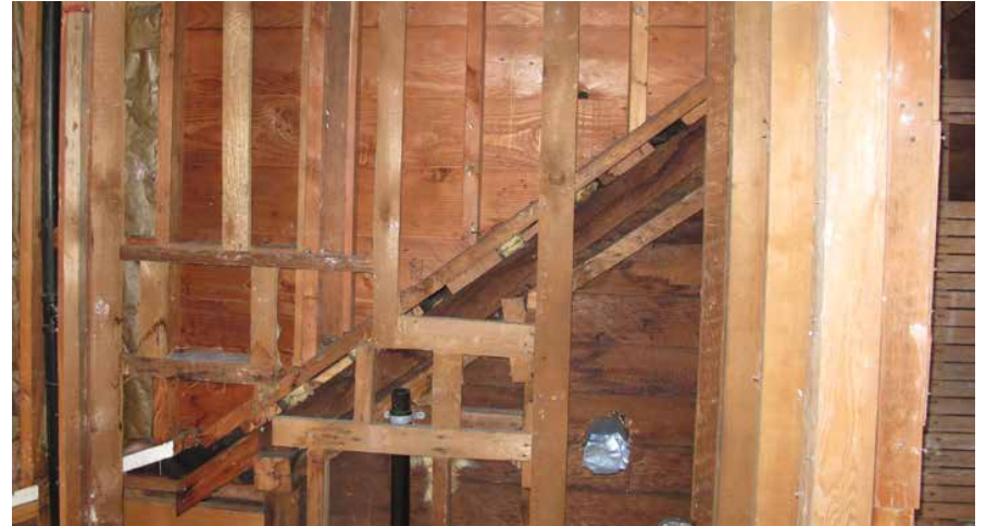
Although the roof framing has been cut out in several locations, virtually all of the planking that formed the exterior soffits were left in place, and can be traced on the east and west sides of the house.
