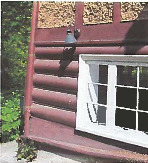
Typical condition of foundation, as seen from the southwest corner of the historic house.
