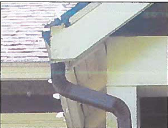
Cross-gabled roof structure of the Sutherland House (top); exposed roof rafters and nailing boards (middle); and typical condition of roof drainage (bottom)
