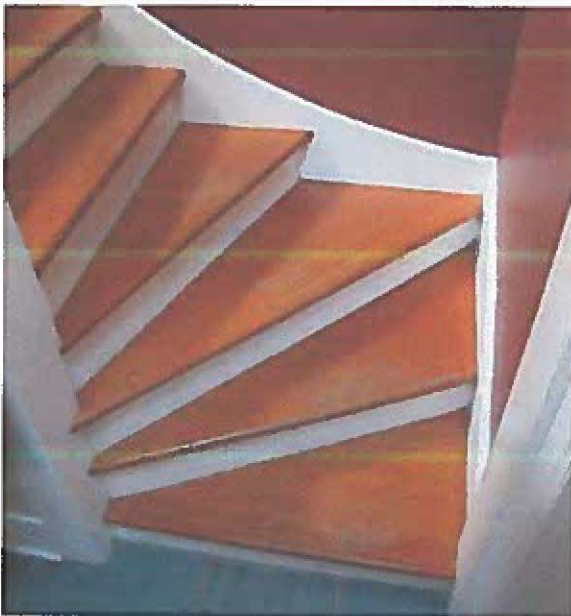
Photos showing newel post (top) and configuration of main staircase with winders (bottom).
