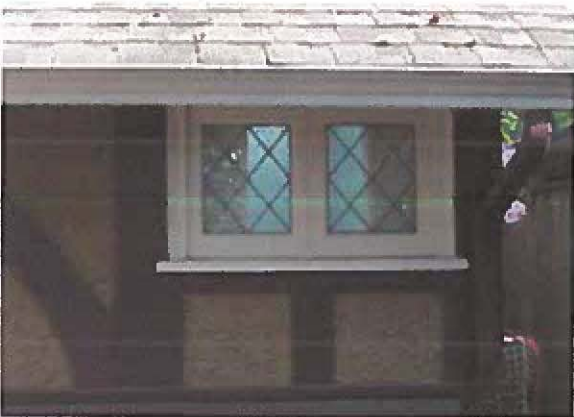
Photos showing typical condition of extant exterior wood windows in different configurations.
