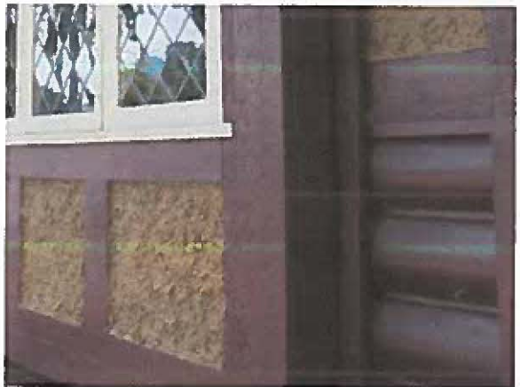
Photos showing typical condition of extant original wood trim work of the historic house, as seen from the ground.
