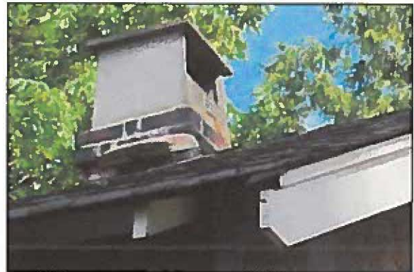
Existing rectangular chimneys: chimney with metal flashing above roof ridge of side-gable (top); and brick chimney with metal chimney cap above roof line to the south.
