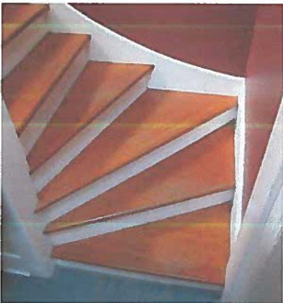
Photos showing newel post (top) and configuration of main staircase with winders (bottom).
