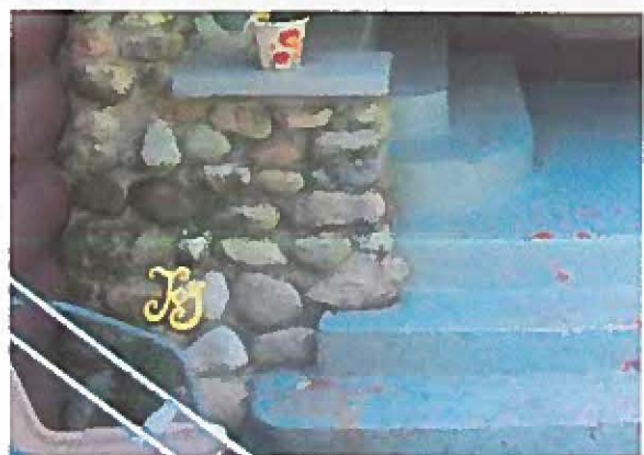
Photos showing typical condition of extant original side-entry porch and stairs of the historic house. Note the crack along the mortar, which also shows biological growth.
