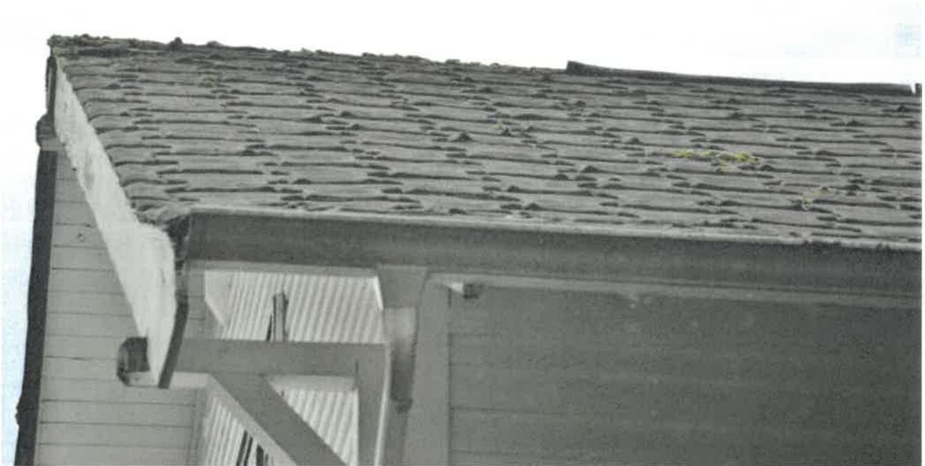
Figure 21: Vintage asphalt roofing with gable end bargeboard and knee-bracket on the left and eavestrough on the right
