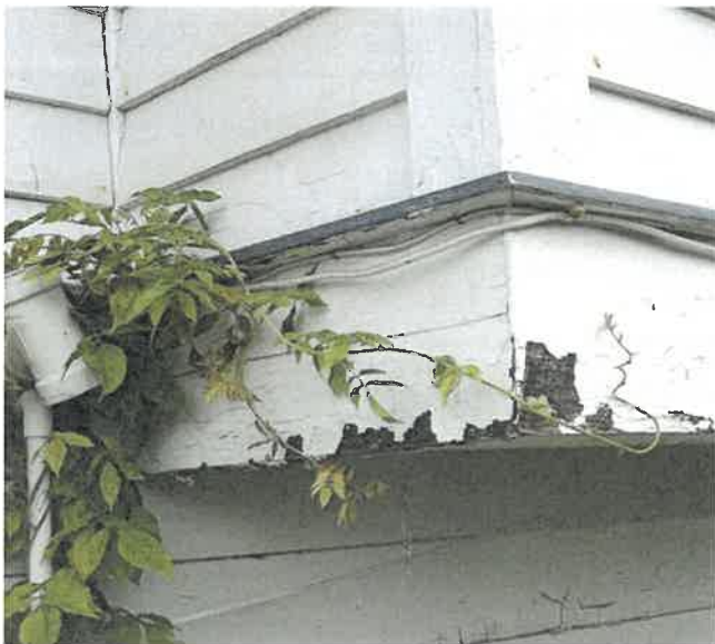
Figure 63: Peeling of siding paint and vegetal invasion
