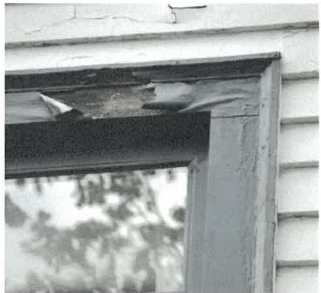
Figure 64: Peeling of window trim paint
