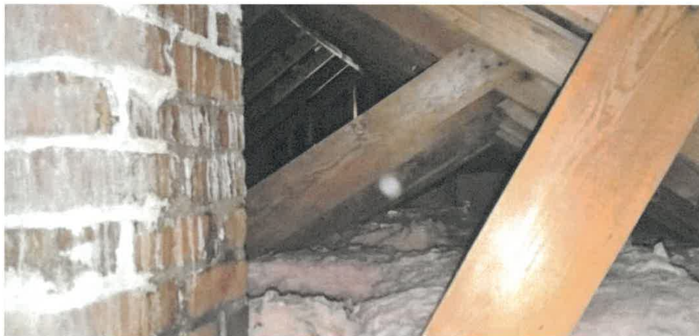
Figure 60: Chimney through attic space, with wooden trusses and bat insulation on above ceiling
